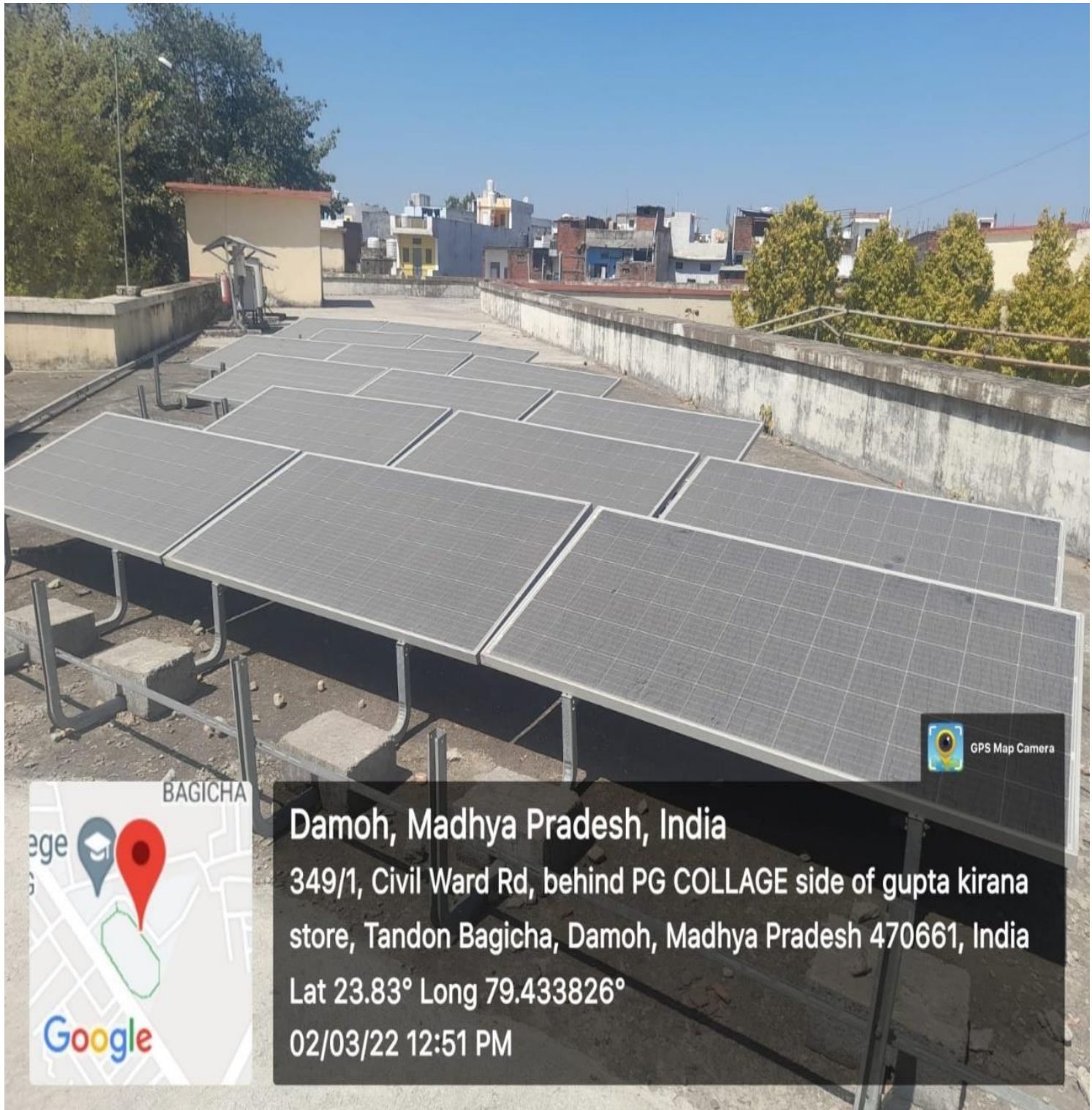
Roof Top Solar Panels Installed on College Building
